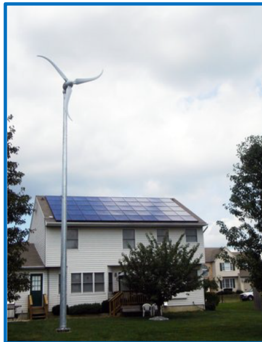
Figure 15. Southwest Windpower's 1.8-kW Skystream wind turbine in a Residential Application
