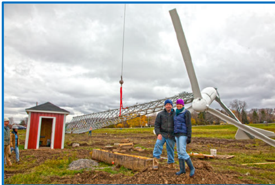
Figure 2. installing a Bergey 10-kW turbine on 120' SSL tower in Lockport, New York.
